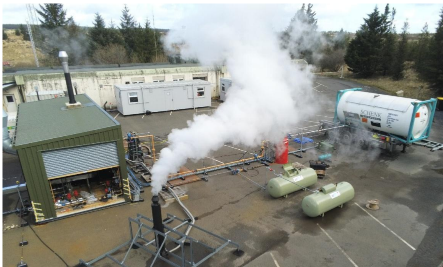
Steam successfully generated by the ammonia-fed steam boiler, pictured during Stage 2 testing of the Amburn project
